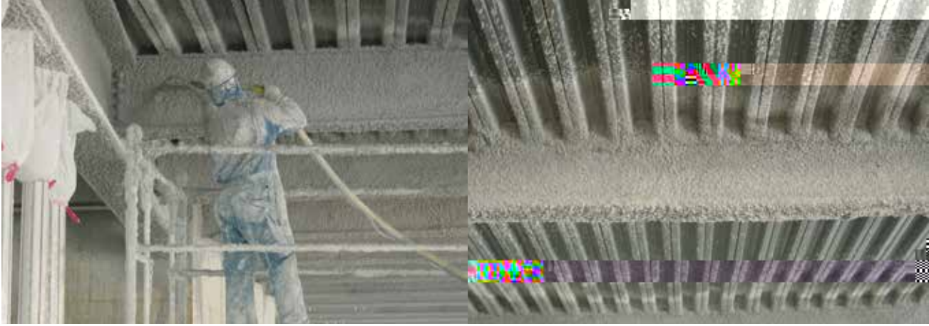
▲ The two-hour assembly ratings in UL Design D982 can be used with any UL-certified spray-applied fire-resistive material (SFRM) with thickness “sufficient to provide a one-hour Unrestrained Beam Rating.”
