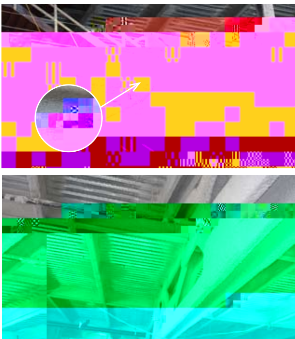
Figure 1: SFRM is applied to steel members to provide fire resistance. The top image shows a thick, textured SFRM application, while the bottom image shows a smoother, more uniform SFRM application.
